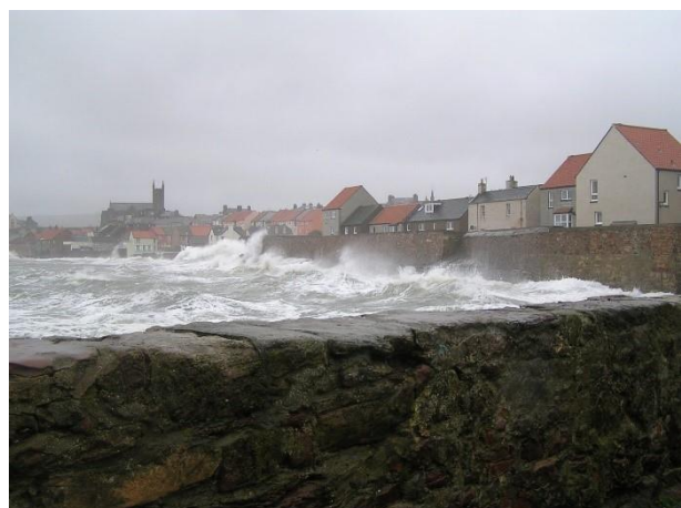
Picture 5.1: Flood damage to properties on Lammer Street, Dunbar, courtesy of Alex
